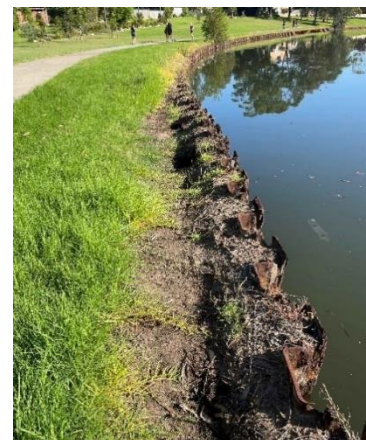
Rusting steel sheet piling and riverbank subsidence at Earlwood presents an immediate danger to the public
